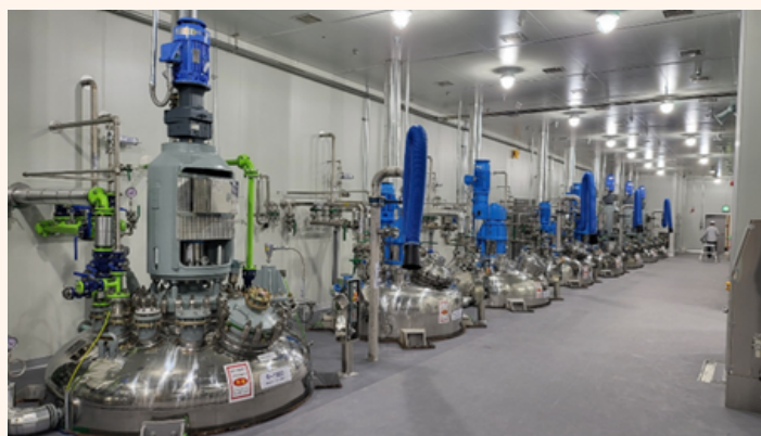
ADC linker component facility in Korea
